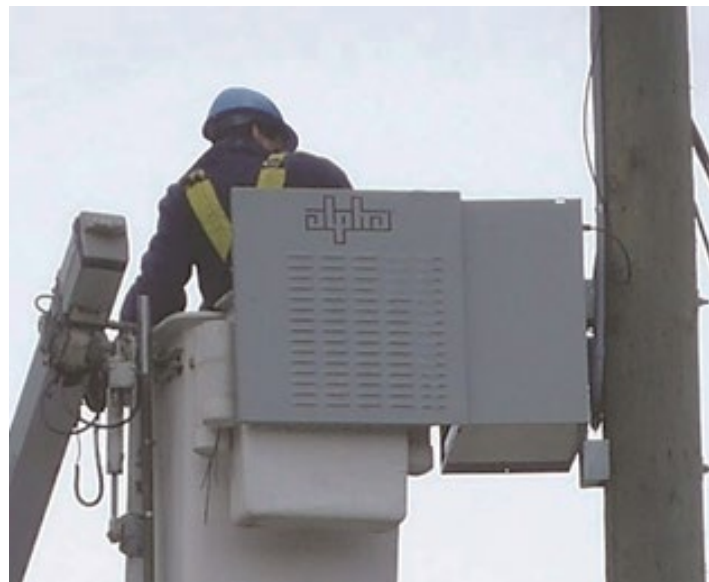
Figure 2 - Pole Mounted Broadband Power Supply
