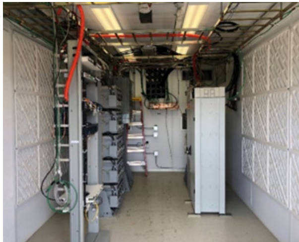
Figure 2 - PCM mounted to interior walls & ceiling of shelter
