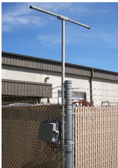
Figure 1 - Transmit antenna for creation of a calibrated leak (image courtesy of Charter).
